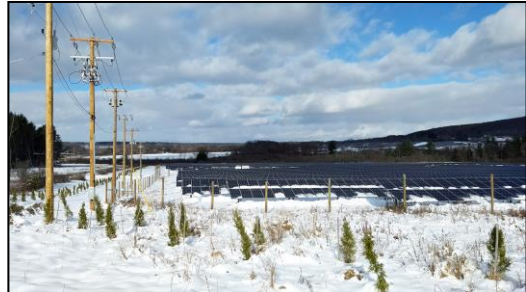
John Mills Electric Large Solar Project in Tompkins County
